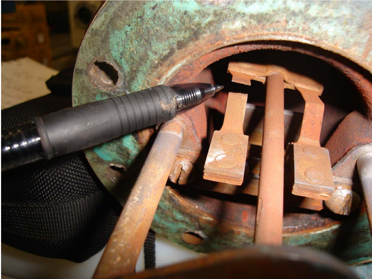
Photo #13 – Bent and Broken Spring on McDonald & Miller (M&M) Series 193-7B Mechanical Combination Low Water Cut-Off/Pump Controller
