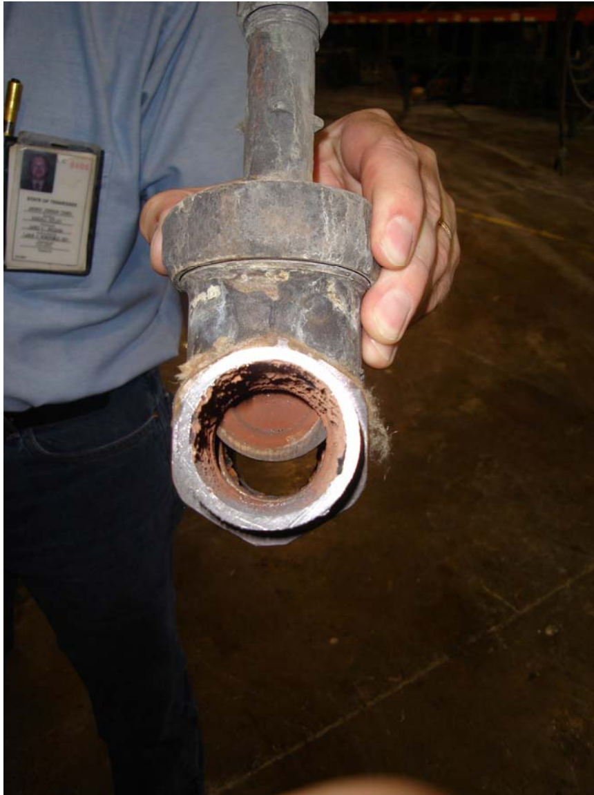
Photo #12 - Bypass to the Modulating Feed Valve. Valve was found in the half open position.
