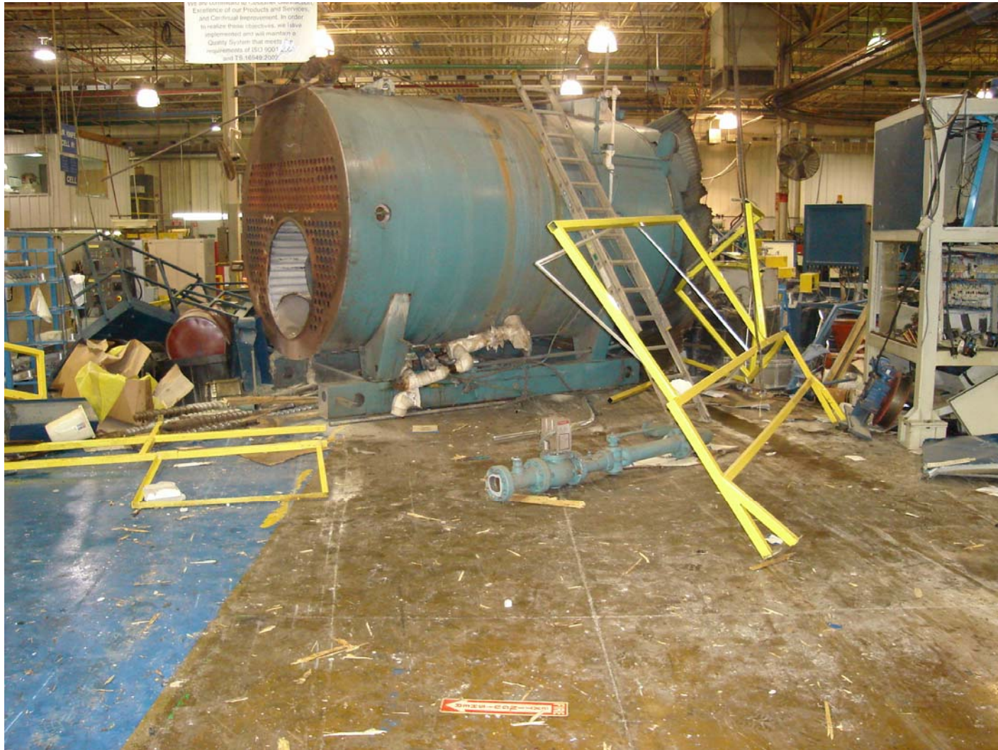
Photo #2 – Final Location of Boiler After Explosion
