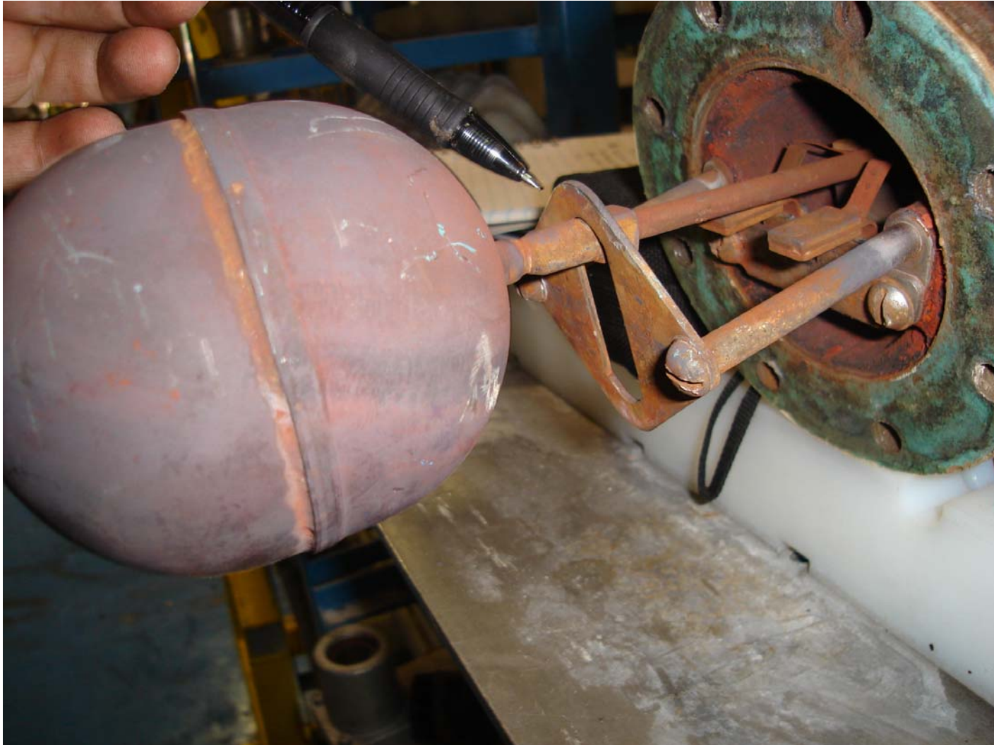
Photo #14 - McDonald & Miller (M&M) Series 193-7B Mechanical Combination Low Water Cut-Off/Pump Controller stuck in the up position
