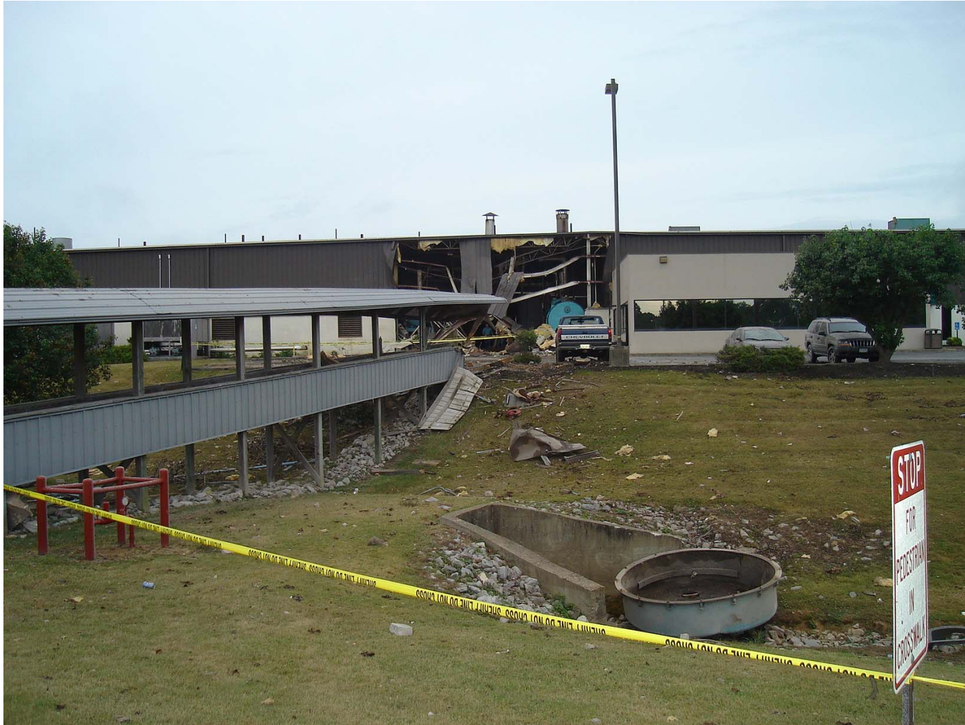
Photo #7 – View of East Wall from Outside Plant (Note Rear Boiler Door in Ditch)
