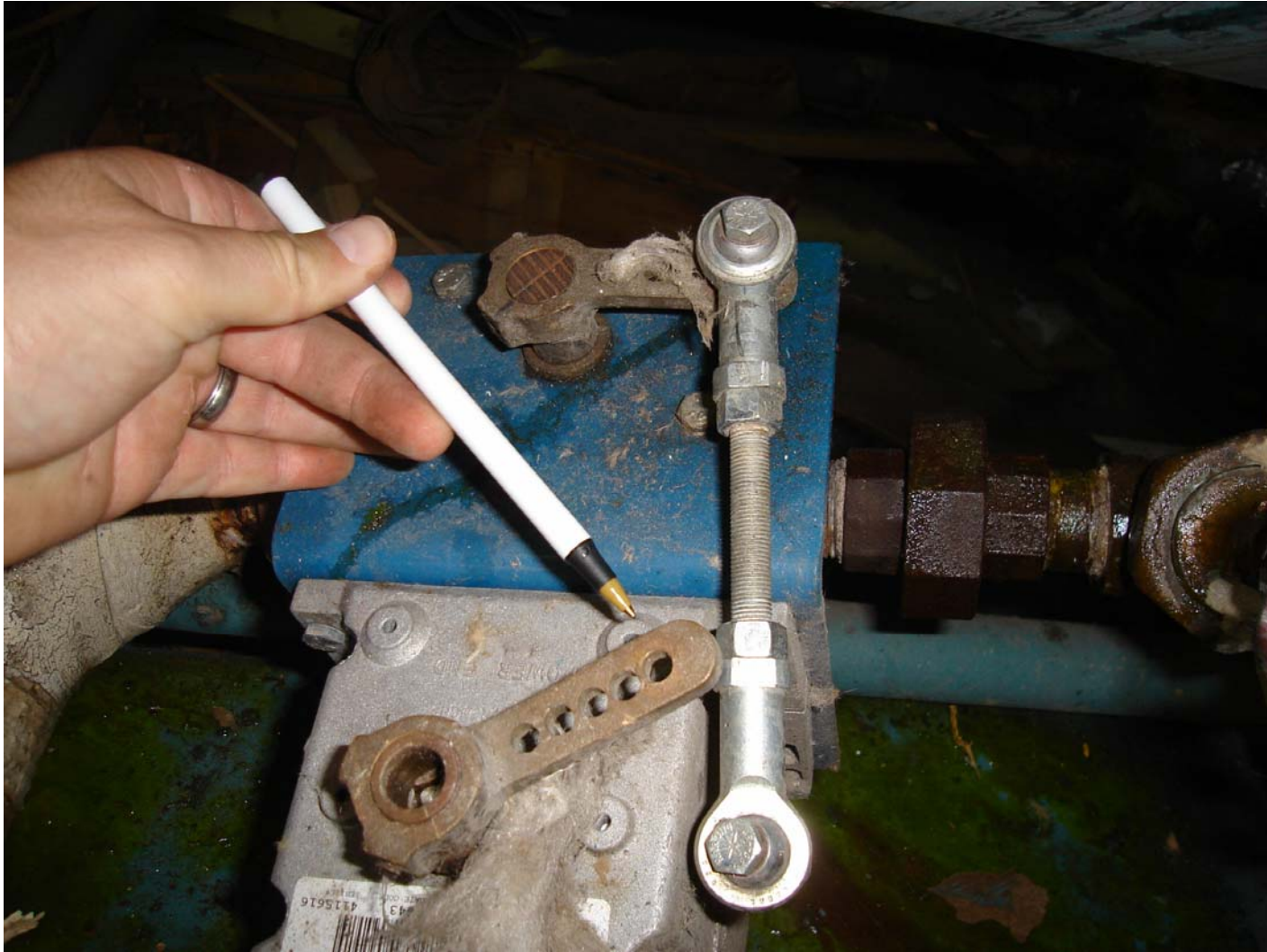
Photo #11 – Modulating Feed Controller and Valve with Disconnected Operating Arm
