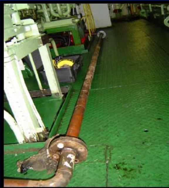
Discharge to Overboard Valve
