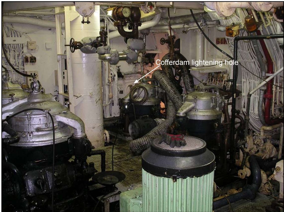
The purifier room
