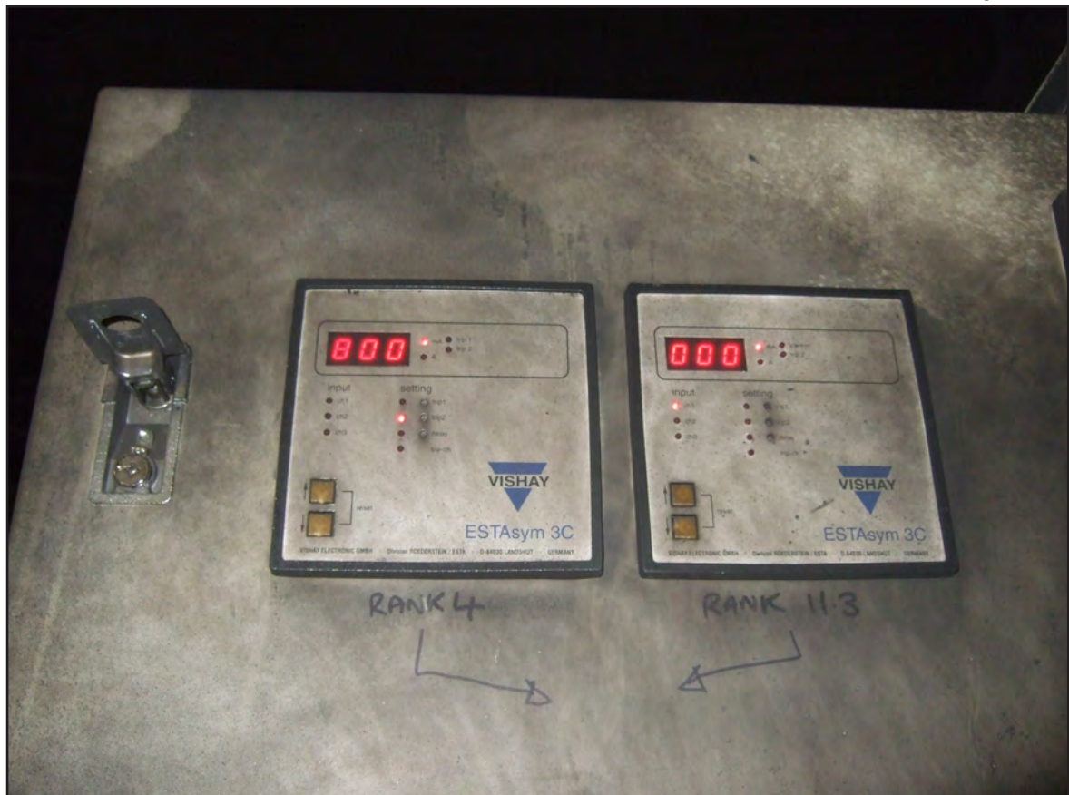
Current imbalance indicators in the aft harmonic filter room
