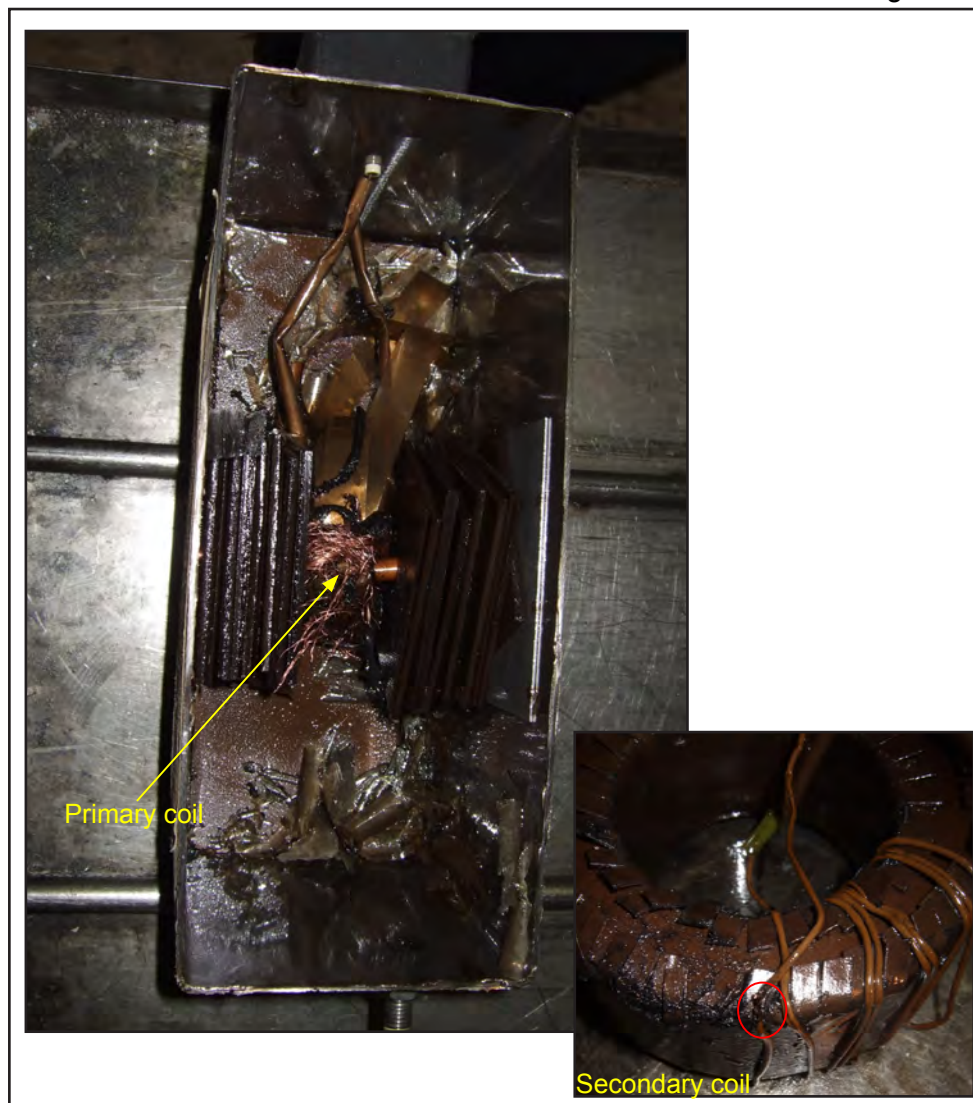
Current transformer for the imbalance detection system with its casing cut open (inset: secondary coil)
