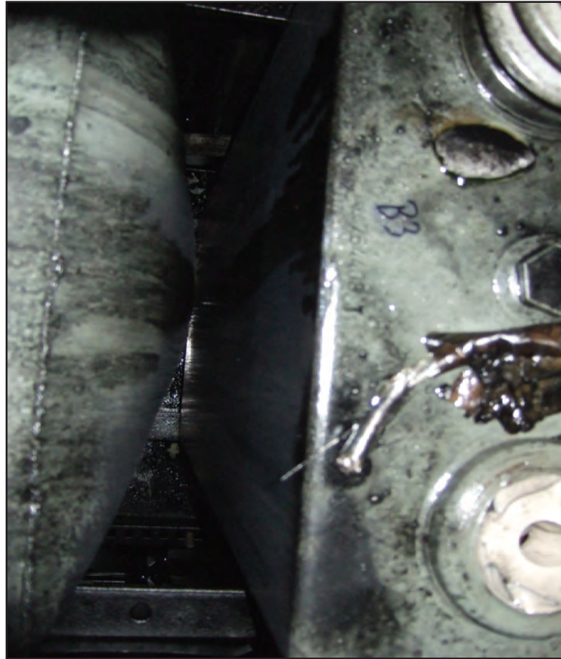
Top view of bulged capacitor
