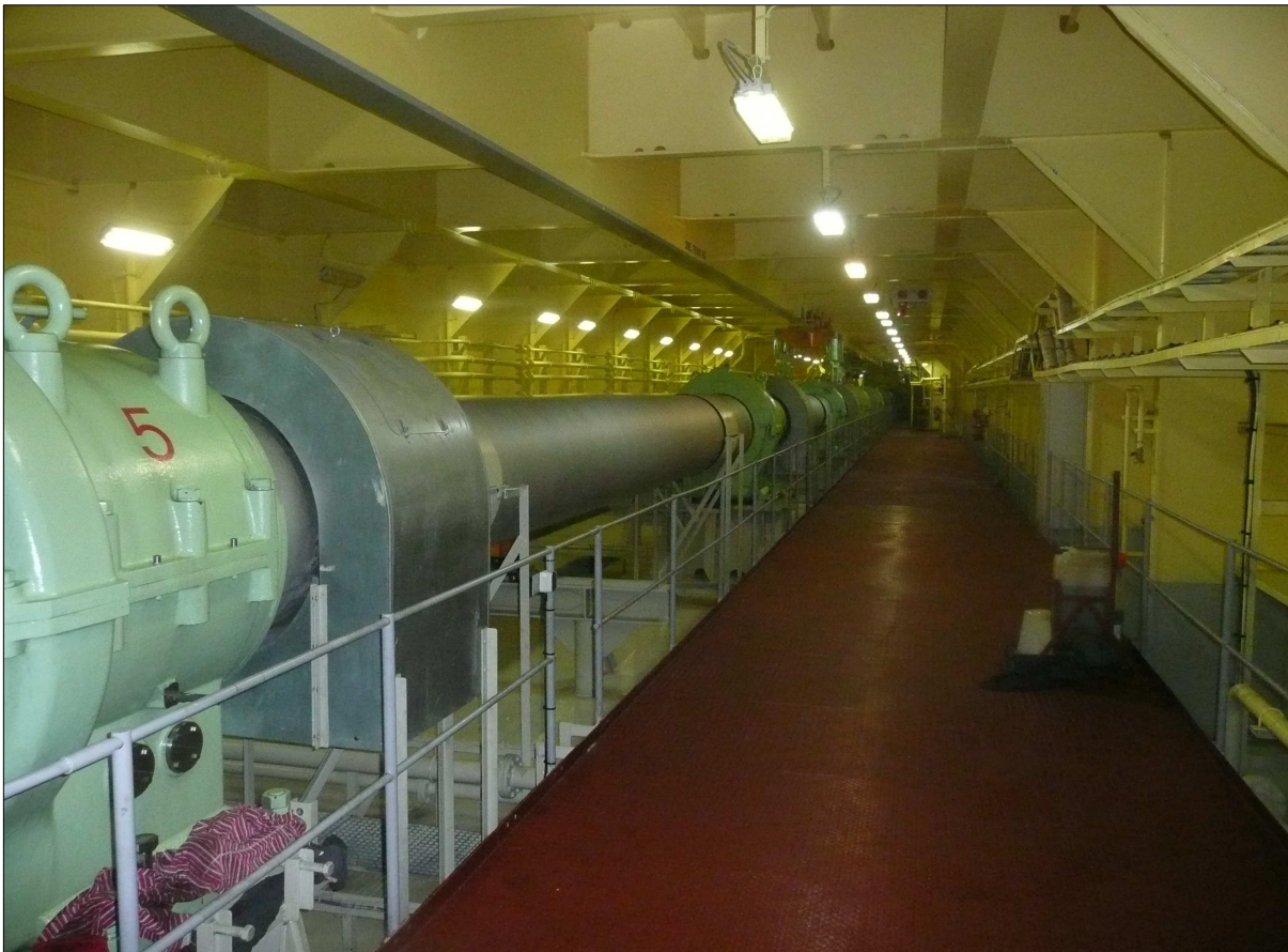
Figure 16: Part of the main propeller shaft tunnel of a sister ship, viewed from fore towards aft Source: DMAIB
