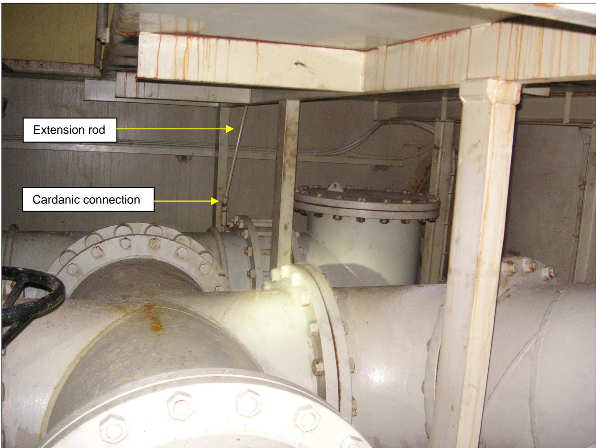
Figure 29: Piping arrangement for cooling water pumps on the tank top in the engine room of a sister ship with extension rod and a cardanic connection in the background Source: DMAIB
