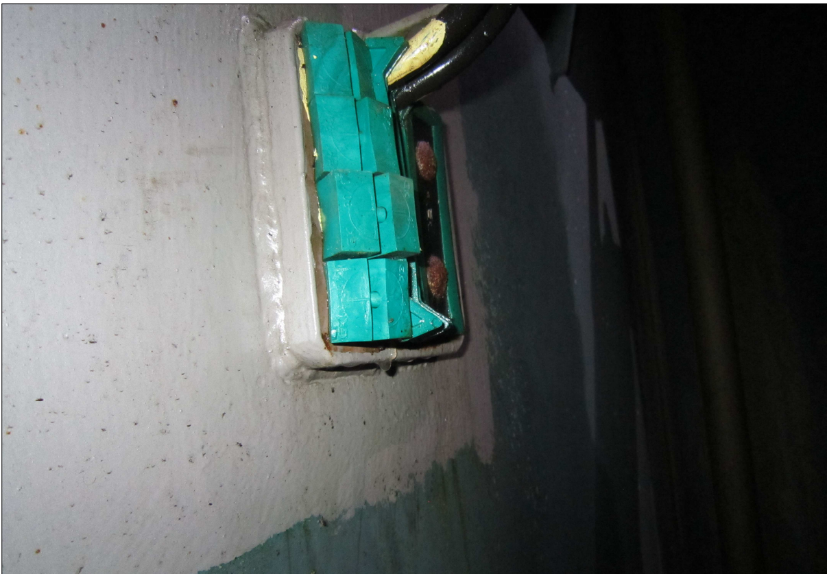
Figure 24: Cable penetration in bulkhead between emergency exit and cargo hold during collapse Source: Maersk Line
