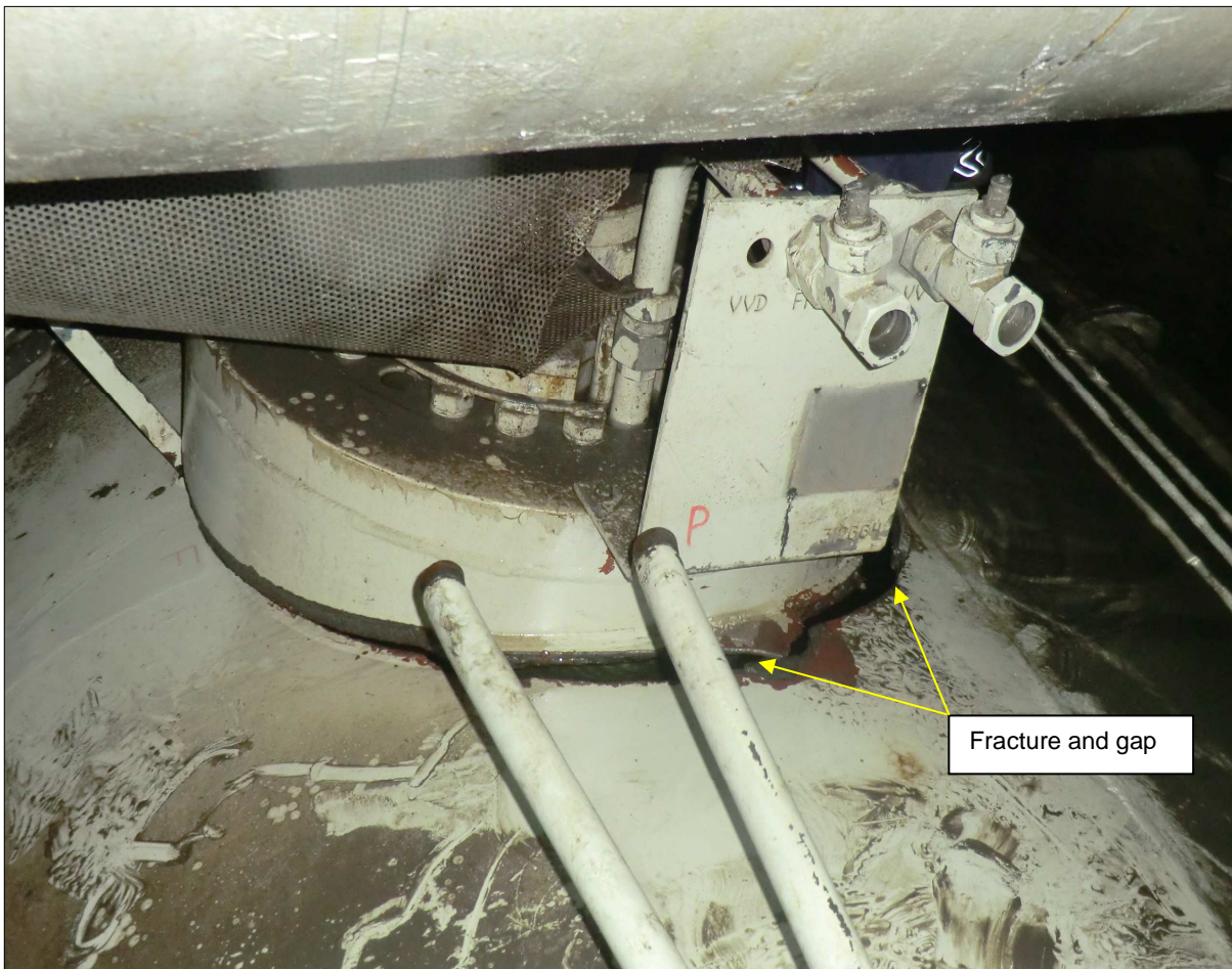
Figure 41: Breakage at the flange neck to the transverse stern thruster tunnel Source: Maersk Line
