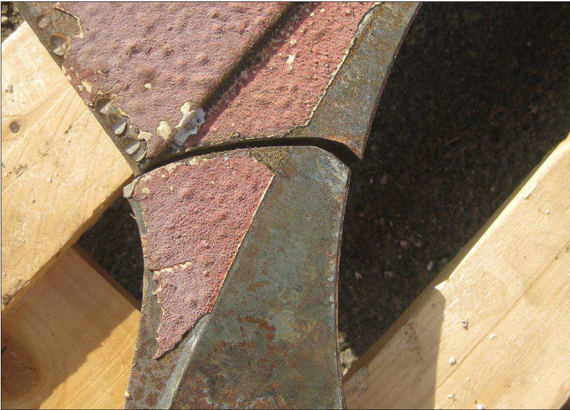
Figure 55: Fracture of supporting base plate for the aft stern thruster Source: BANDAK Engineering/Rolls Royce Marine
