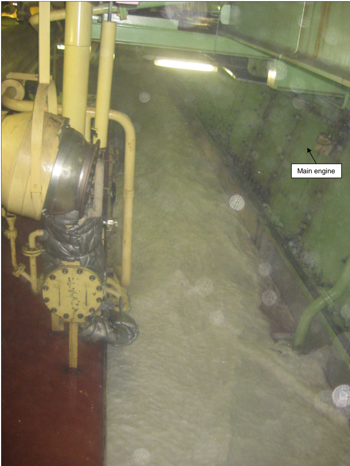
Figure 20: Engine room getting flooded, viewed forward from the aft of the engine room port side Source: Maersk Line
