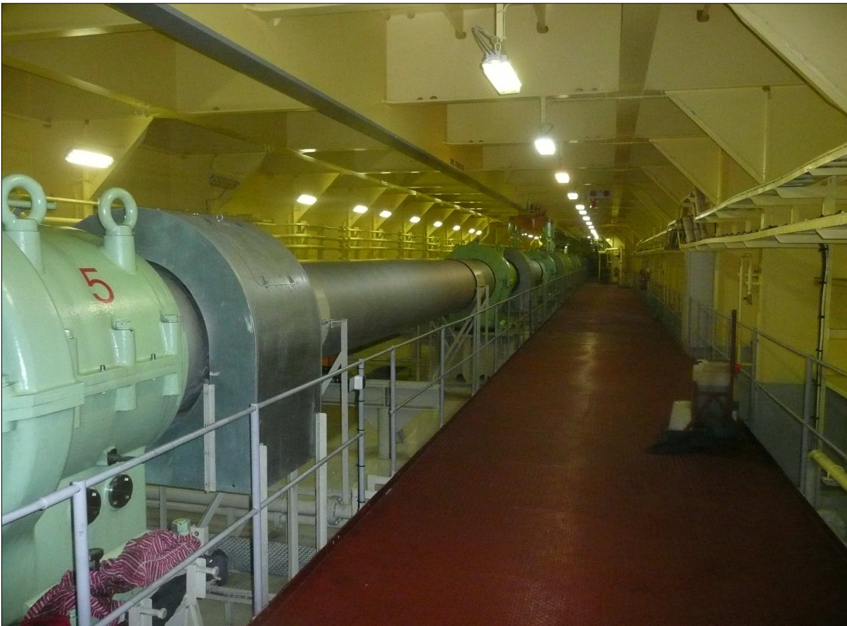
Figure 16: Part of the main propeller shaft tunnel of a sister ship, viewed from fore towards aft Source: DMAIB
