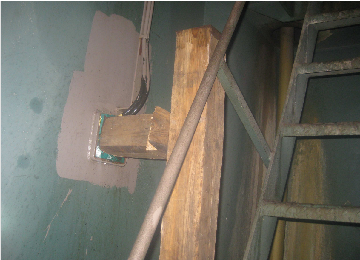
Figure 25: Temporary repair of cable penetration in bulkhead between emergency exit and cargo hold Source: Maersk Line
