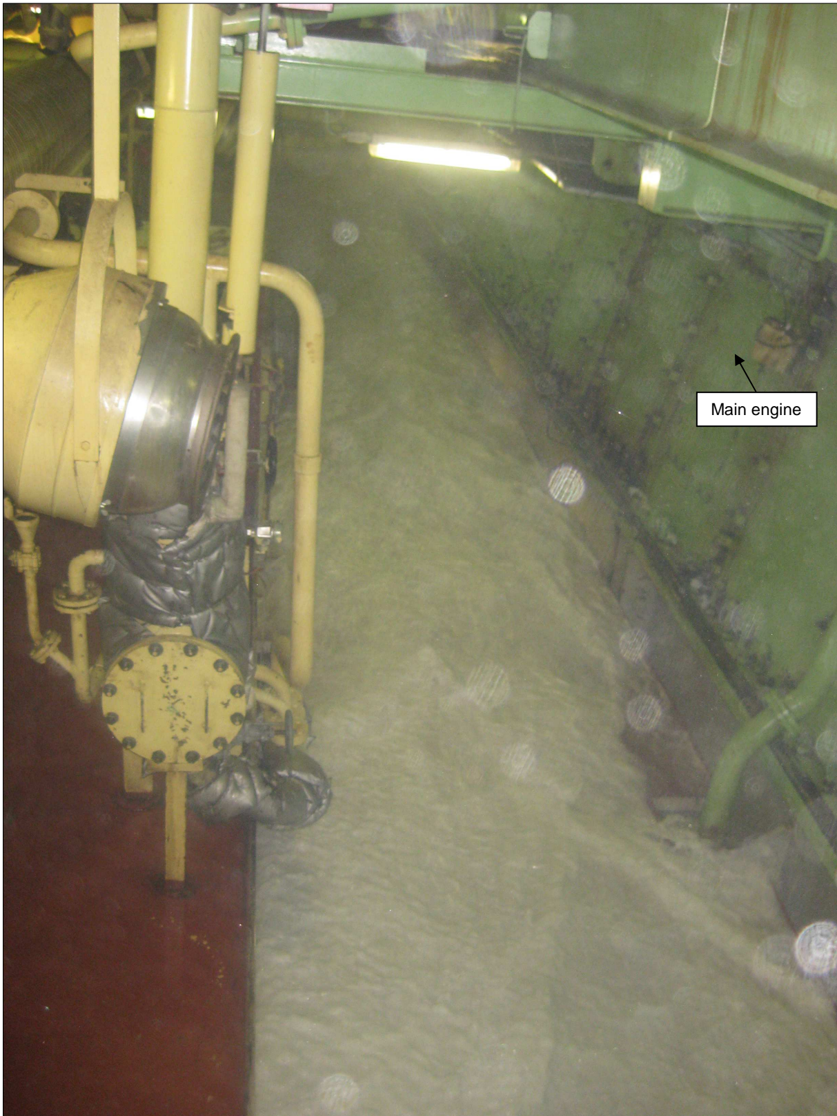
Figure 20: Engine room getting flooded, viewed forward from the aft of the engine room port side Source: Maersk Line
