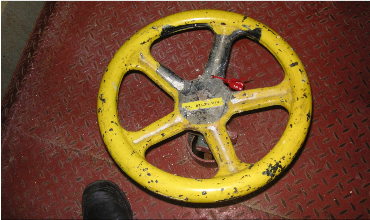
Figure 28: Handwheel for emergency direct suction from the engine room by the largest seawater pump of a sister ship Source: DMAIB
