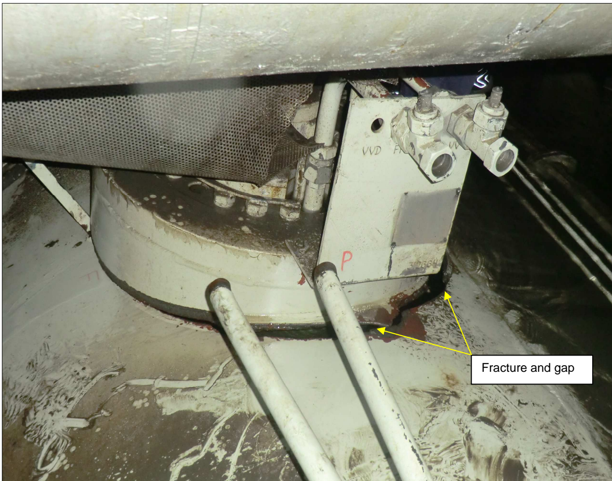
Figure 41: Breakage at the flange neck to the transverse stern thruster tunnel Source: Maersk Line
