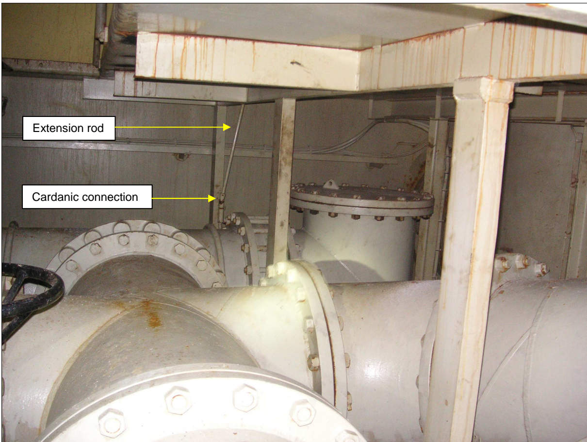
Figure 29: Piping arrangement for cooling water pumps on the tank top in the engine room of a sister ship with extension rod and a cardanic connection in the background Source: DMAIB
