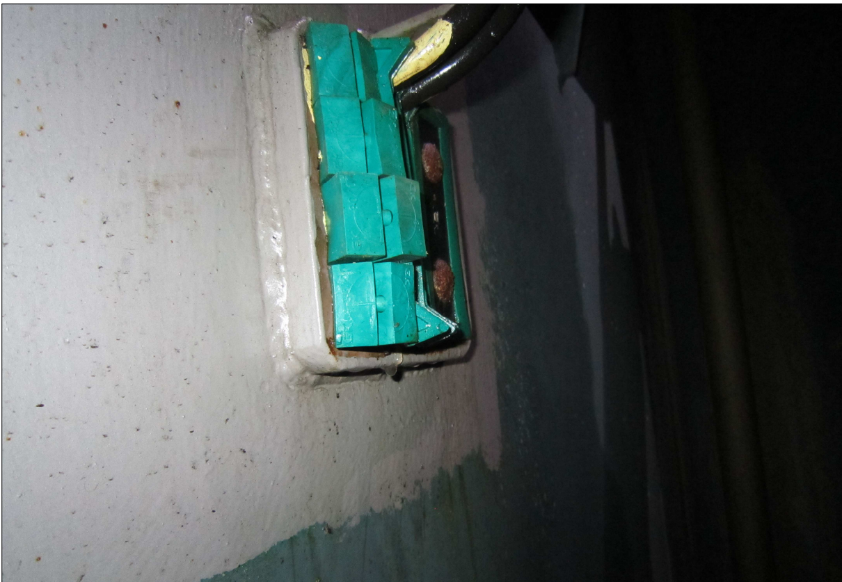
Figure 24: Cable penetration in bulkhead between emergency exit and cargo hold during collapse Source: Maersk Line
