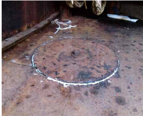
Photo 3. Silicon sealant on 1 of the 26 hatch covers
