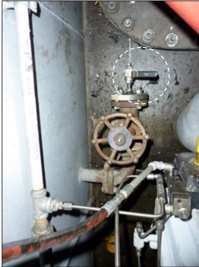
Photo 2 - No. 1 Day Tank Stbd Drain
