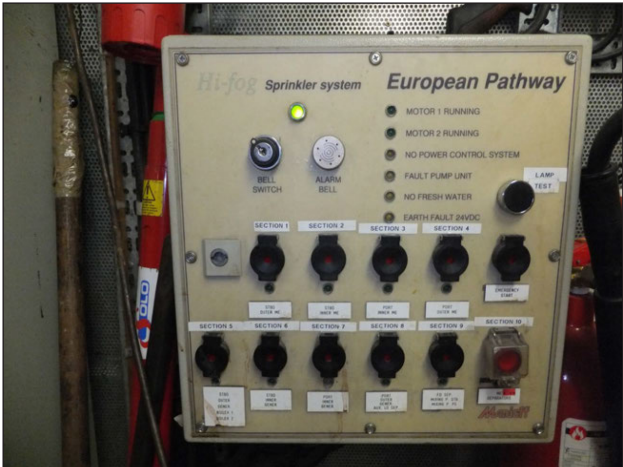
Figure 7: Hi-fog control panel in engine control room ( Pride of Canterbury was previously named European Pathway )
