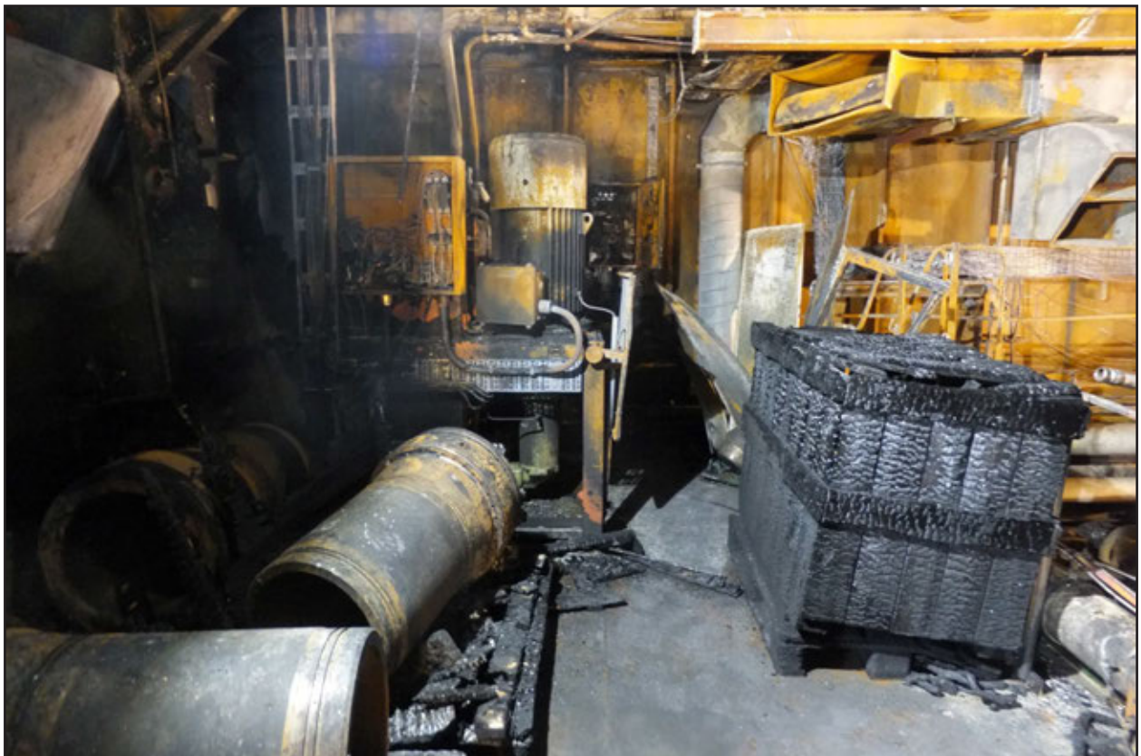
Figure 11: Fire damage looking aft on starboard side, deck 2
