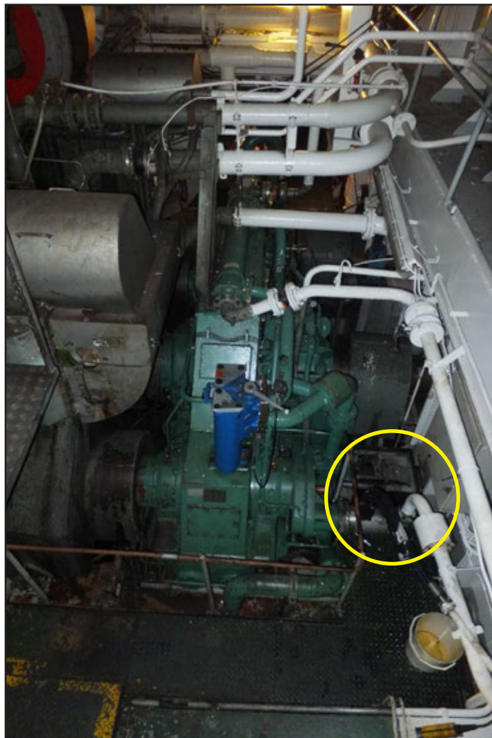
Figure 14: Power take-off controllable pitch propeller pump, deck 1
