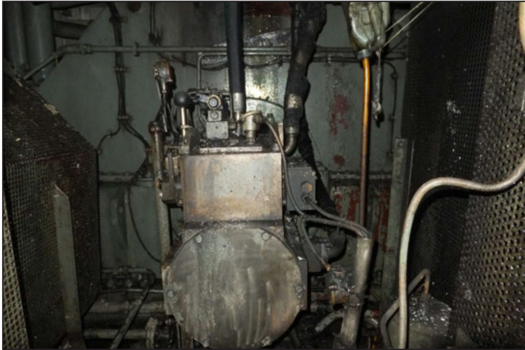
Figure 13: Oil distribution box, deck 1
