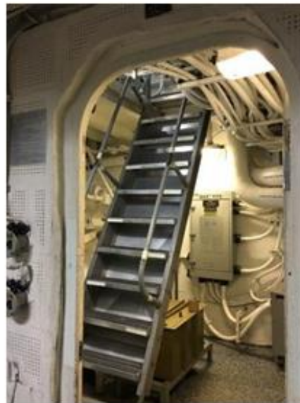
Figure 9 – Non-watertight door frame from Berthing 2 to the ladder going up to Berthing 1 Access Trunk. There is no hatch at the top of this ladder to prevent water from flooding up into Berthing 1.
