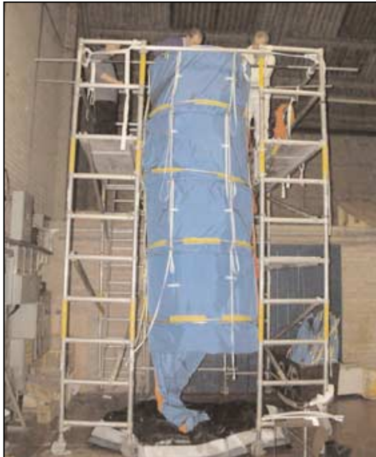
Four cells rigged up in RFD's factory for the reconstruction
