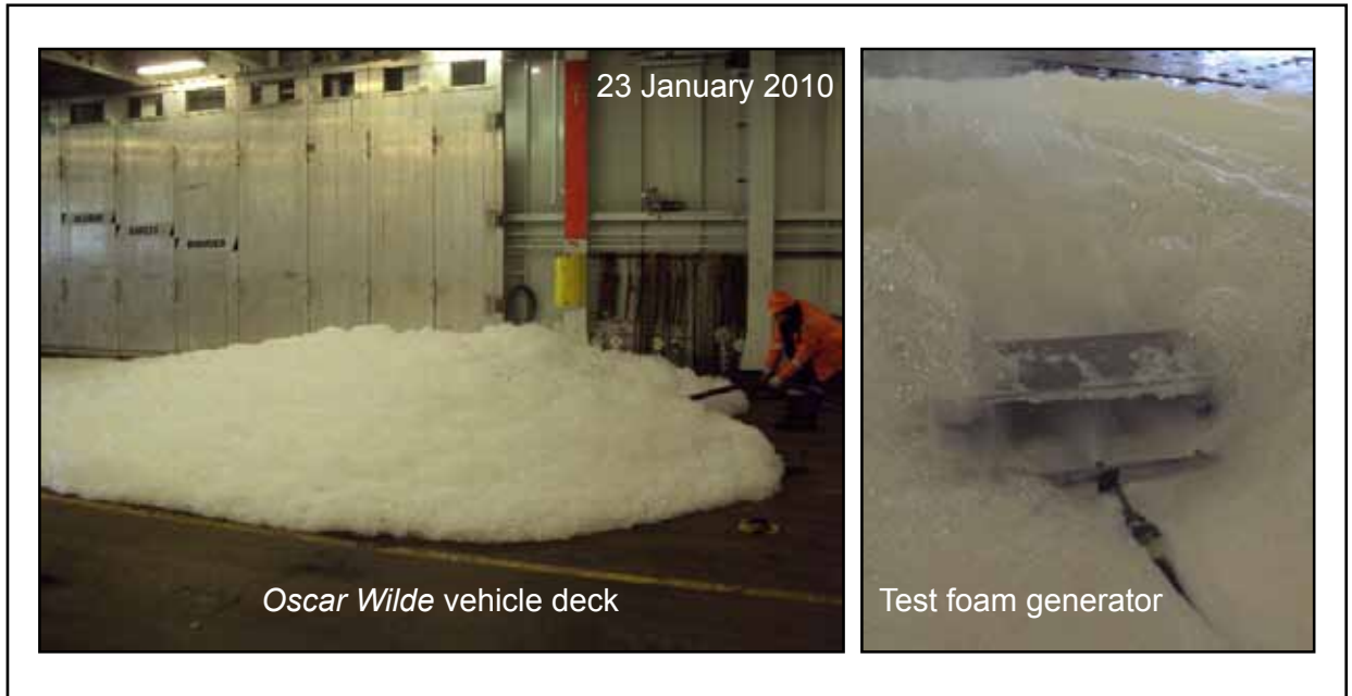
Hotfoam system discharge test
