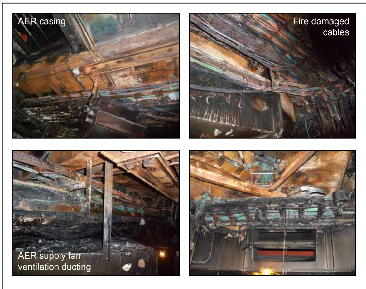
Fire damage to deckhead cables in the auxiliary engine room
