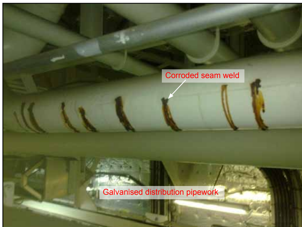
Hotfoam system survey on other vessels
