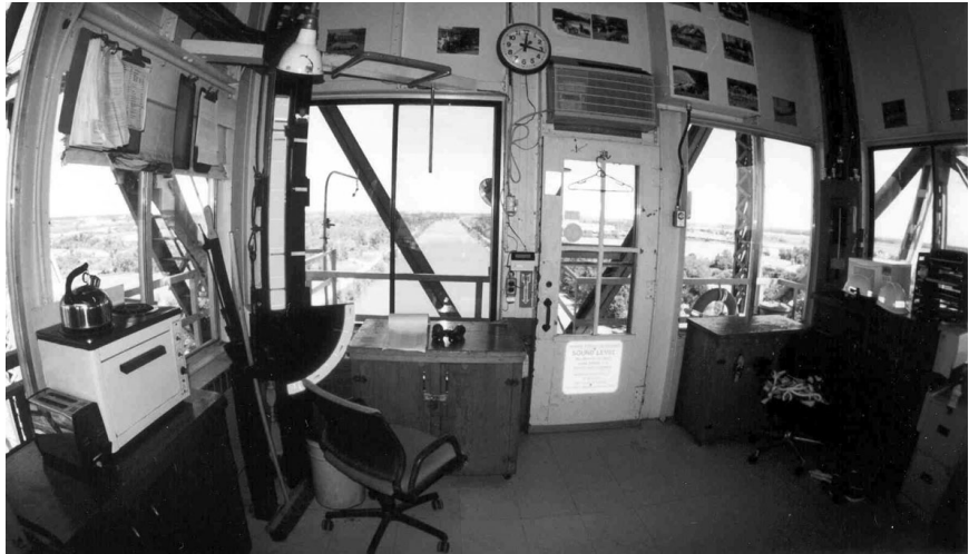
Photo 6. Looking north from inside bridge operator control room with bridge in fully raised position (using fish-eye camera lens).
