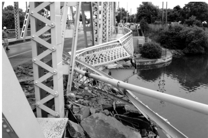
Photo 5. Damage to Bridge 11. (Photograph by Thorold Fire Department)
