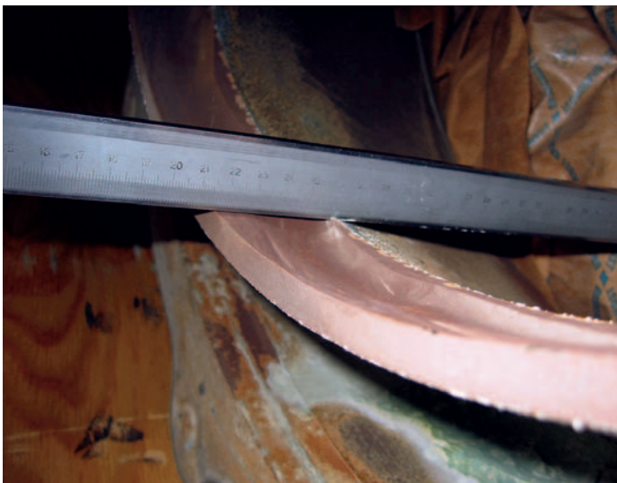
Worn turbine diffuser.
