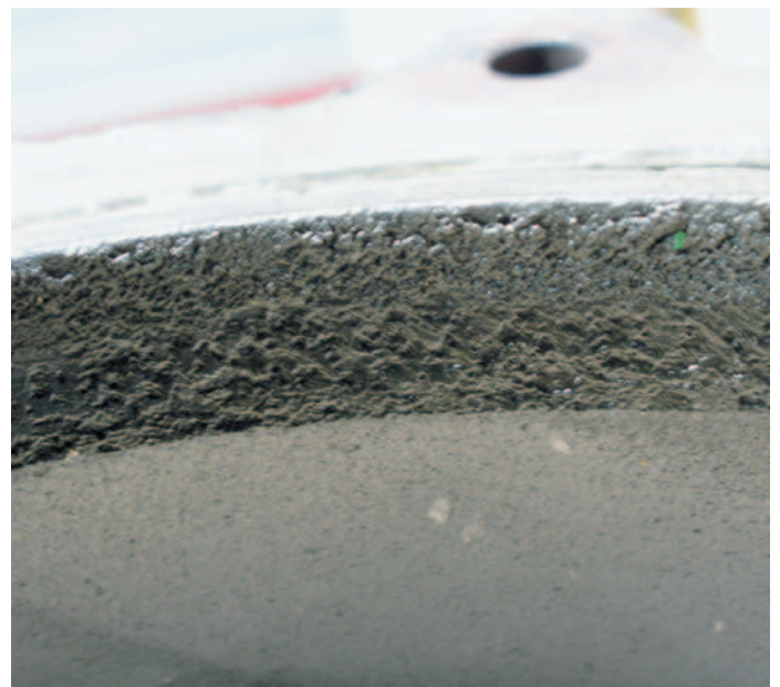
Layer of scale deposited on a turbine diffuser
