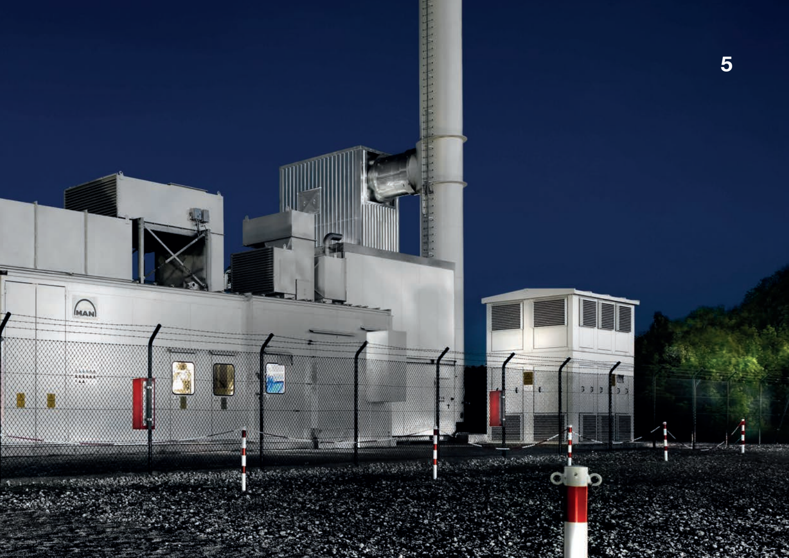
Solvay GmbH's gas turbine plant in Rheinberg operates a MAN MGT6000
