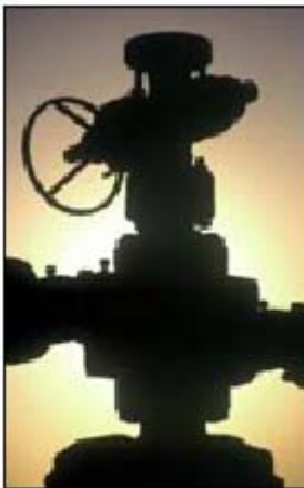
A Natural Gas Wellhead
