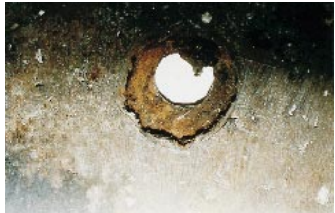
Figure 6.2 Bilge main perforations of pipewalls due to SRB corrosion
