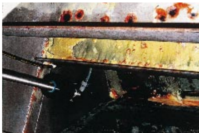
Figure 7.5 Storage tank contamination indicating biofilms and SRB pitting corrosion
