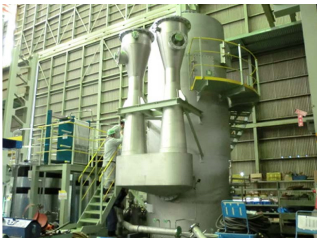
Figure 4 IGS type scrubber (Front) Venturi (Rear) Cleaning tower
