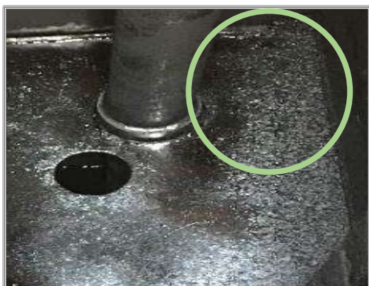
Sedimentary oil sludge at the edge of tank / between the floor space and wall surface.
