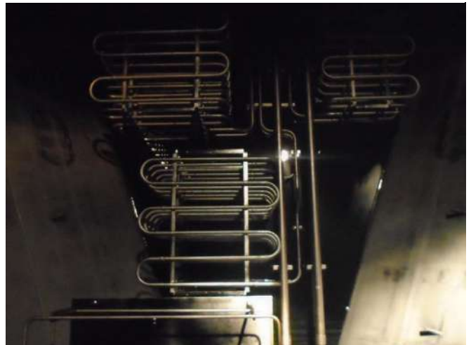
4. Heating coils close-up
